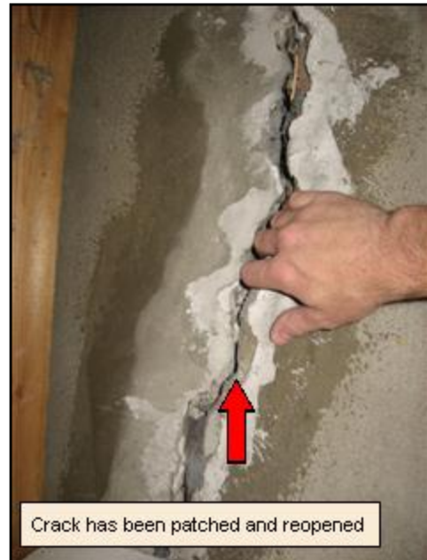
5. Cracked foundation wall
