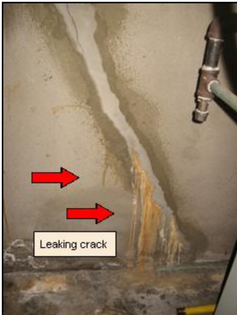
4. Foundation crack - leaking
